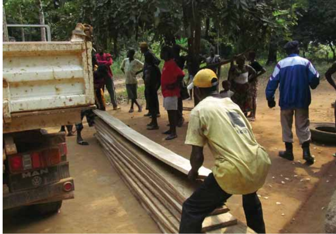
Residents of Tumba Village off loading building supplies for Tumba Primary School construction
